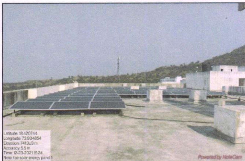
Photograph of Roof Top Solar PV Plant:
