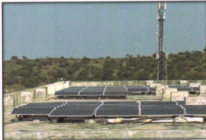
Photograph of Solar PV Plant:
