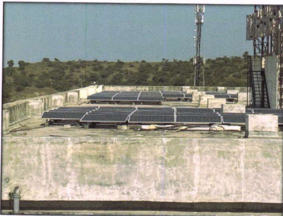
Photograph of Solar PV Plant:
